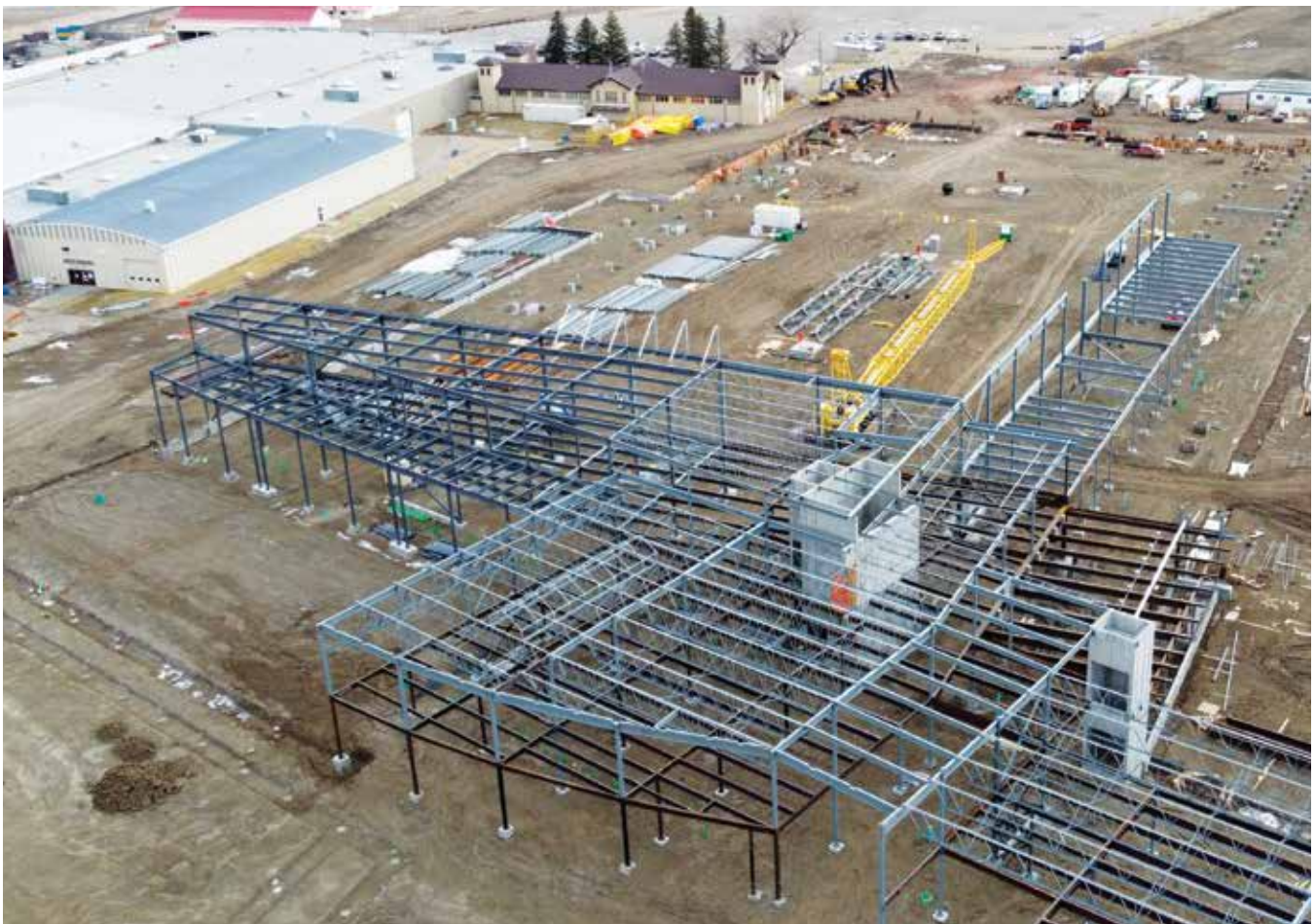
Construction continues at Exhibition Park, the new Agri-Food Hub is expected to be completed in 2023. PHOTO COURTESY OF EXHIBITION PARK LETHBRIDGE.
