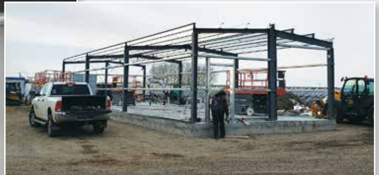
Spark Power O & M Building Nitro Construction Ltd.
